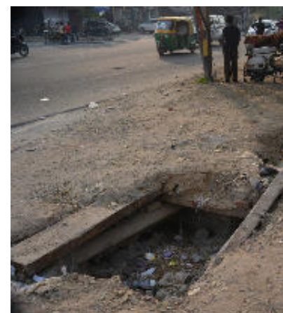
Clogged stormwater drain
